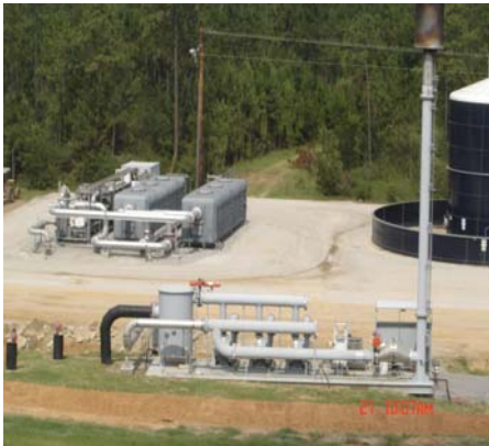
LFG Flare System and Treatment Unit Located at the Pecan Grove Landfill Property
