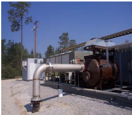
LFG Flare System and Treatment Unit Located at the Pecan Grove Landfill Property
